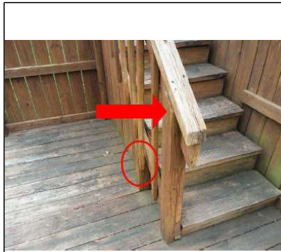
Loose railing and spindle
