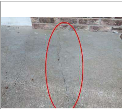
Typical cracks at porch
