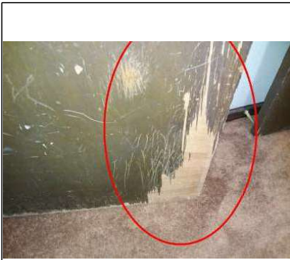
Damage on interior garage door
