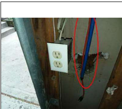
Front hose bib supply line
