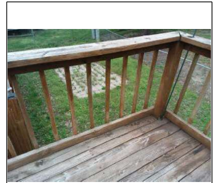
Large openings in railing
