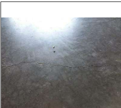
Garage floor cracks
