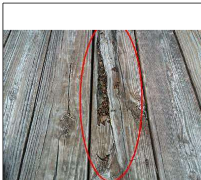
Wood rot at deck
