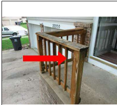
Porch railing loose
