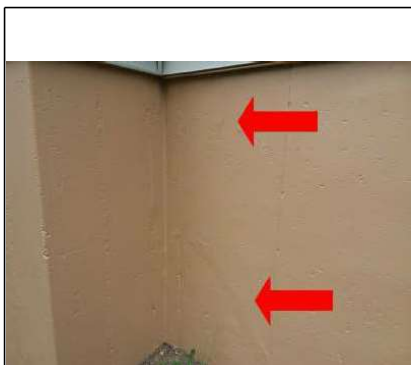
East exterior wall cracks
