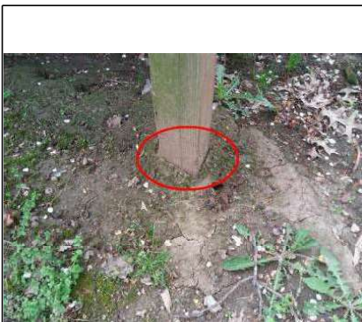
Deck post below soil
