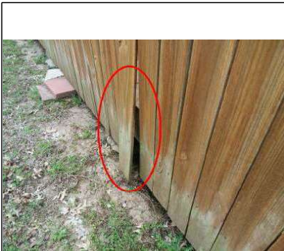
Loose board at pool fence
