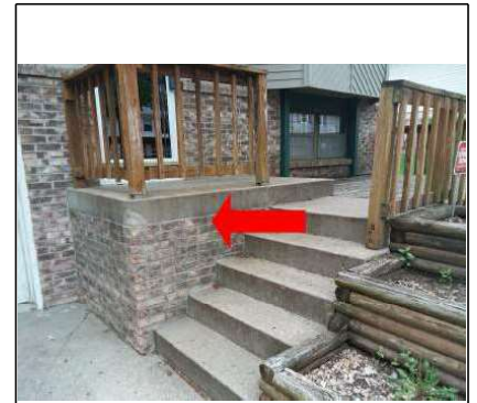
Porch railing needed
