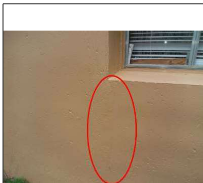
East exterior wall cracks
