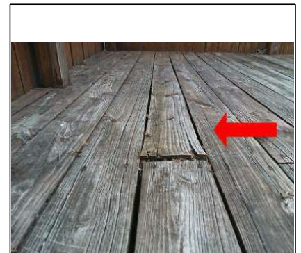
Loose boards at deck
