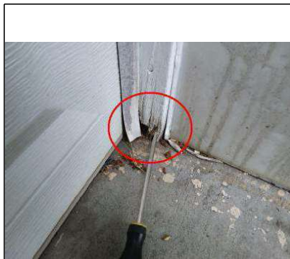
Garage frame wood rot
