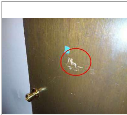
Damage on basement door
